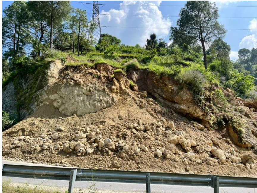
Figure 12. Photograph showing a landslide at stop-5. Here, the lithology comprises the Infra-Krol limestone as encountered at stop-3 east of Narendra Nagar.
